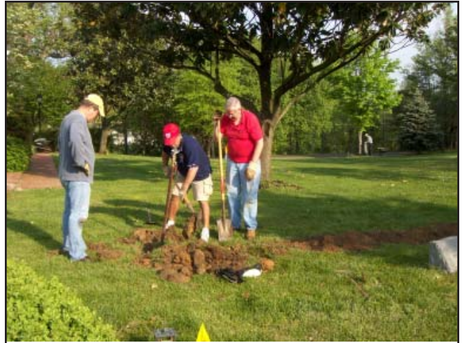
OK, where's the leak?
